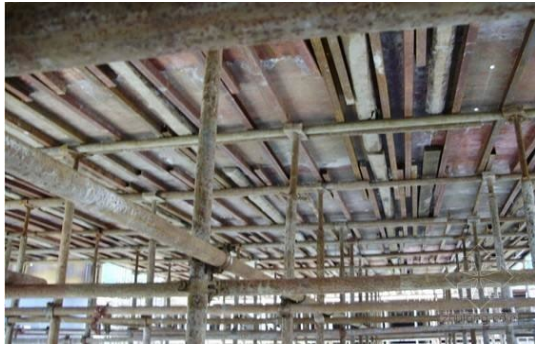
a) Real-site scene of safety hazards of scaffolding
