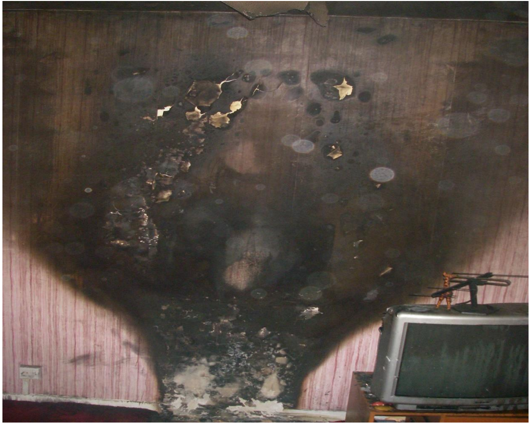
Figure 3.14. Pattern of burning to wall surface behind refrigerator
