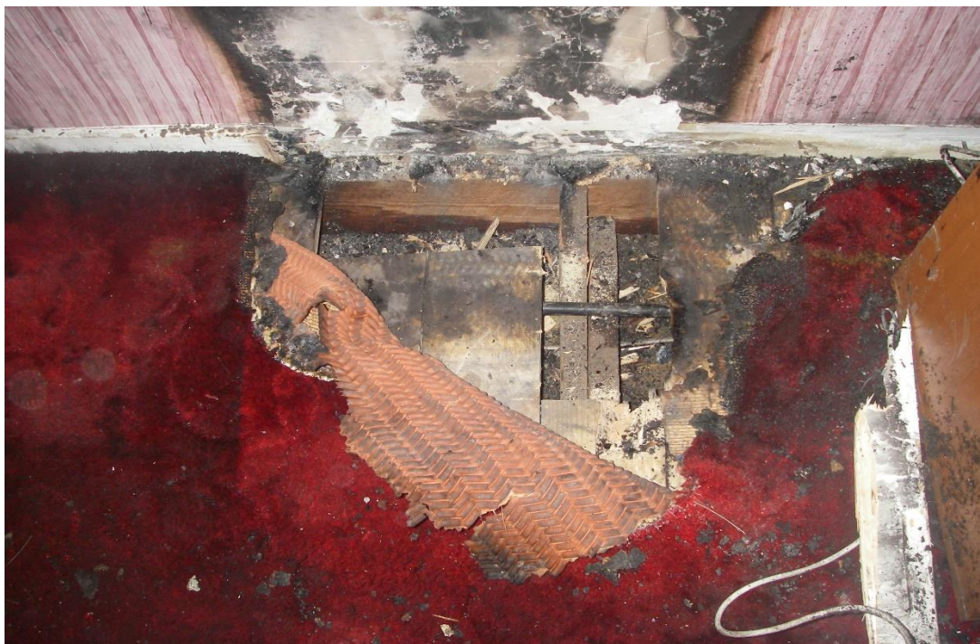
Figure 3.13. The floor beneath the refrigerator has been removed to check for any fire spread and confirms that the fire originated above the floor surface.
