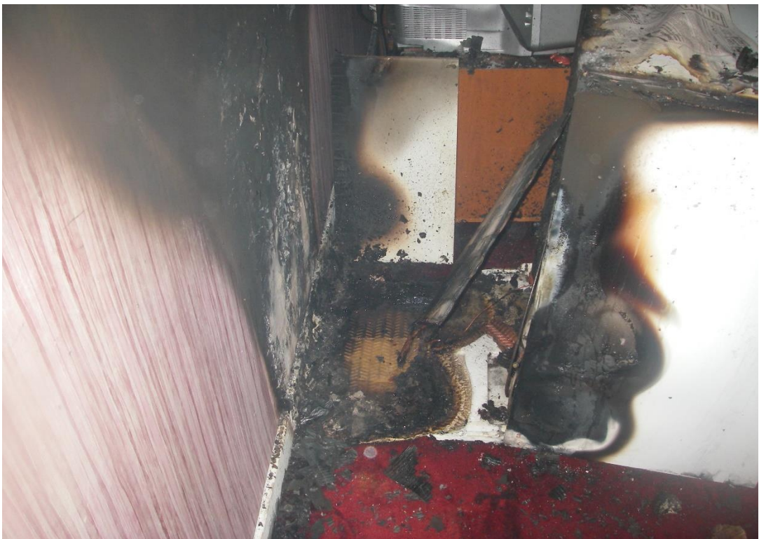
Figure 3.11. The refrigerator has been moved forward to reveal the damage to rear wall surface and floor beneath.
