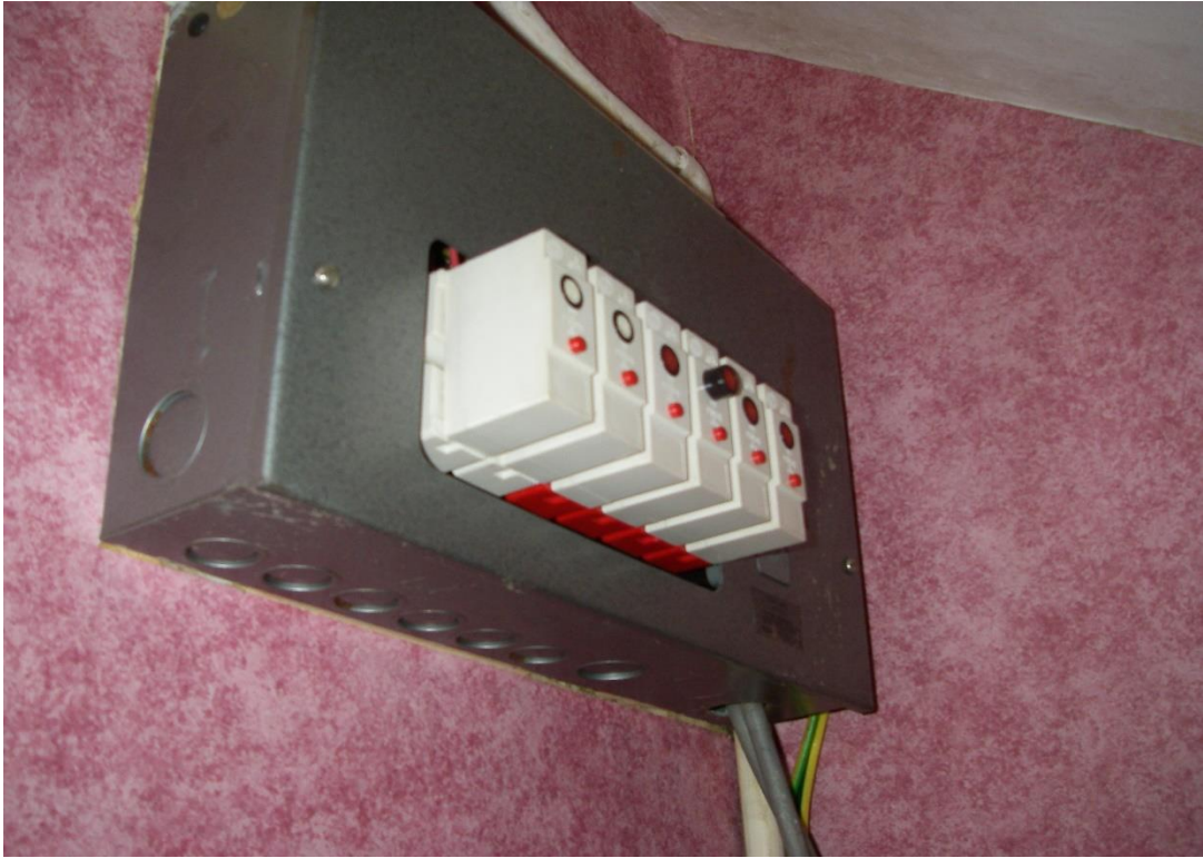
Figure 3.9. Electrical consumer unit showing one circuit breaker operated.
