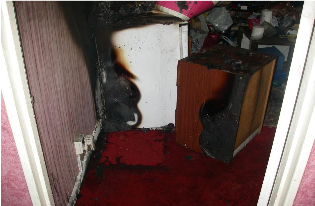
Figure 3.10. The burn patterns observed on the refrigerator and the surrounding objects and surfaces including the adjoining cabinet.
