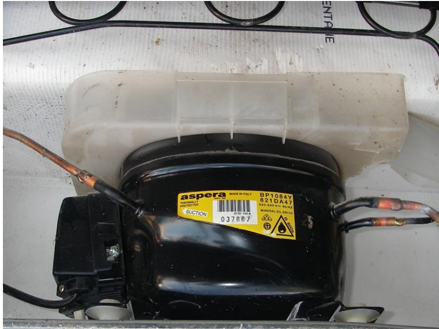
Figure 6.2 An example of an undamaged plastic evaporation tray.
