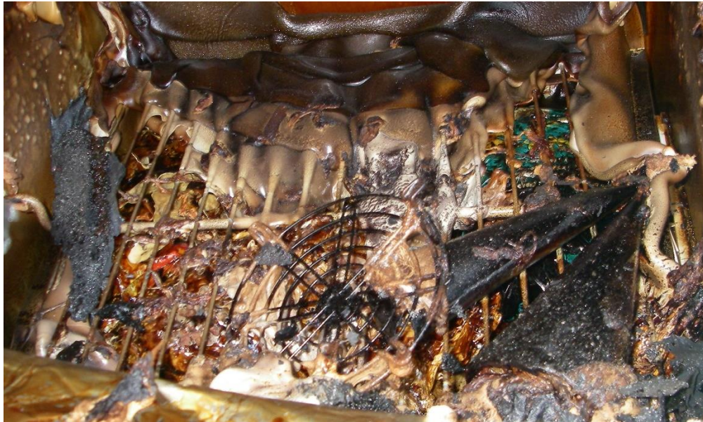
Figure 3.3. Steel fan cover in internal debris (LFB Fire incident 101005091 06/2009)
