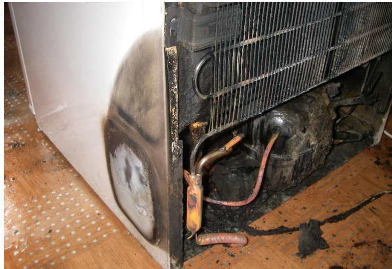
Figure 3.6. Further example of familiar burn pattern. (LFB Fire incident no 77514081 05/2008)
