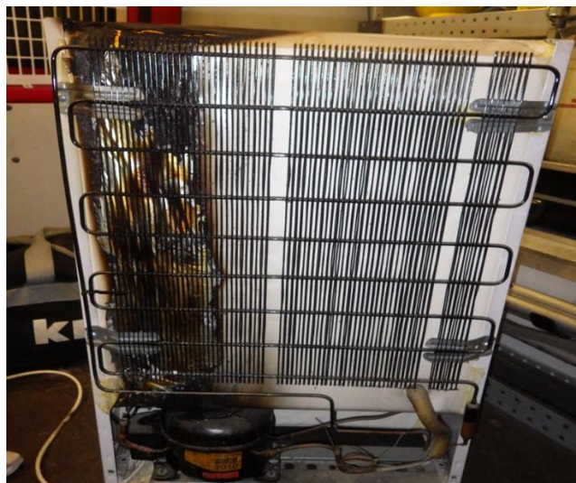
Figure 6.8 An example of flame spread up the rear of a pre-1993 appliance, backed by a plastic film covering metal foil, which has prevented ignition of the foam insulation material. (LFB Fire incident no 10885122 06/2012)
