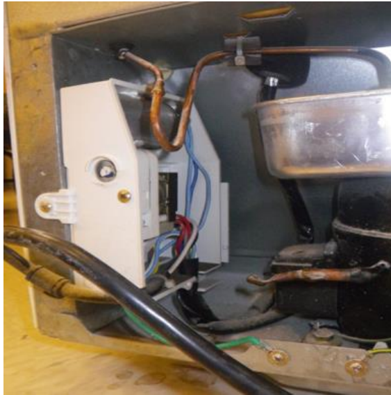
Figure 7.3 An American appliance with both the capacitor and the defrost timer switch mounted in a white fire resisting box within an all metal compressor housing and metal evaporator tray.
