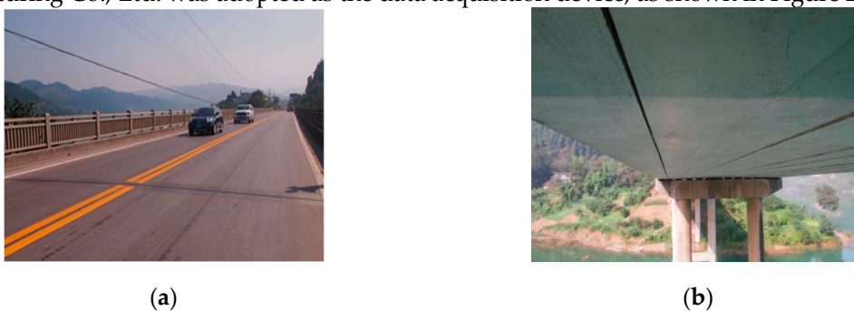
Figure 26. Li ziwan Bridge of Chongqing City: (a) Upper surface; (b) Lower surface.
