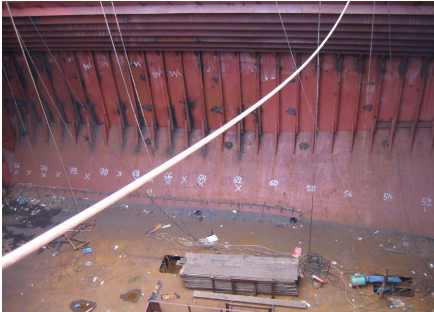
Figure 3. A typical large container hold on a ship. The 3-vehicle CROCELLS prototype is designed to be able to operate between the vertical stiffeners whose separation is 700mm.
