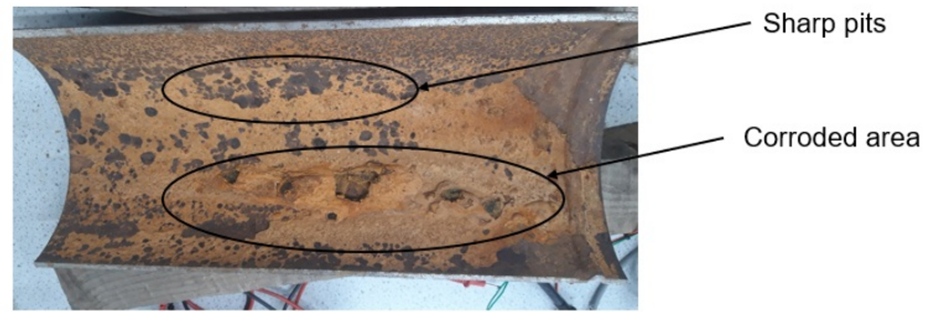
FIGURE 5.8: The image of corroded pipe sample showing the areas with wall thickness loss.
