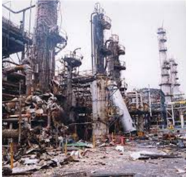
FIGURE 1.3: Humber refinery, United Kingdom, gas plant damage by fire and explosion [27].
