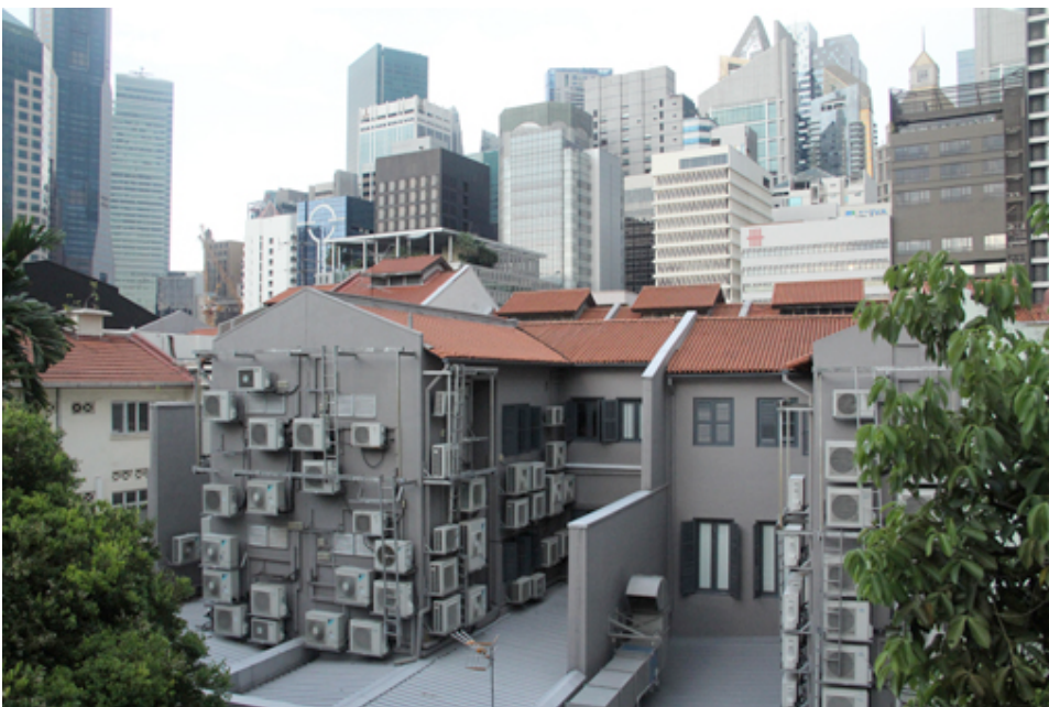
Figure 1. Typical installation of split unit condensers in a crowded and hidden location.
