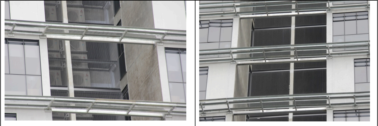
Figure 3: Condenser units with louvers: condensers visible (left) and hidden from view (right).
