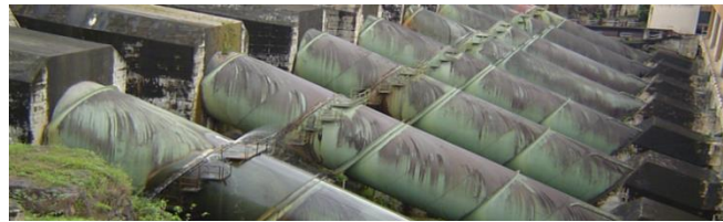
Figure 2.25 Song Loulou hydroelectric power plants Source Eneo/AS Sonel Cameroon (2015)
