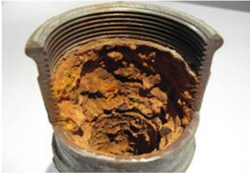
Figure 6: Formation of scale in the pipe (McLay, 2015).
