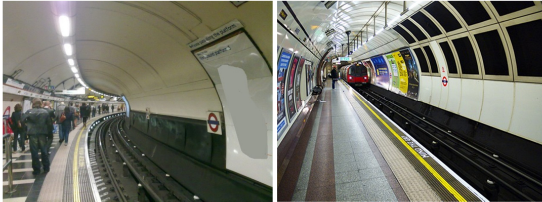
Figure 5:2 Left: Curved platform. Right: platform showing vents outlets and ceiling metal cladding.
