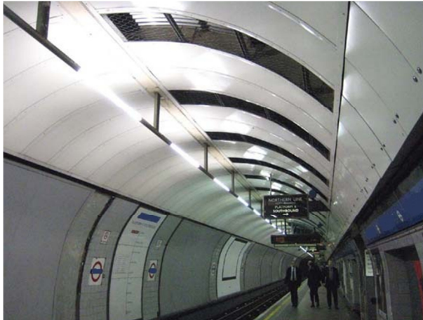
Figure 5:18 Platform ceiling metal clad showing the panel dimensions and air gap depth.
