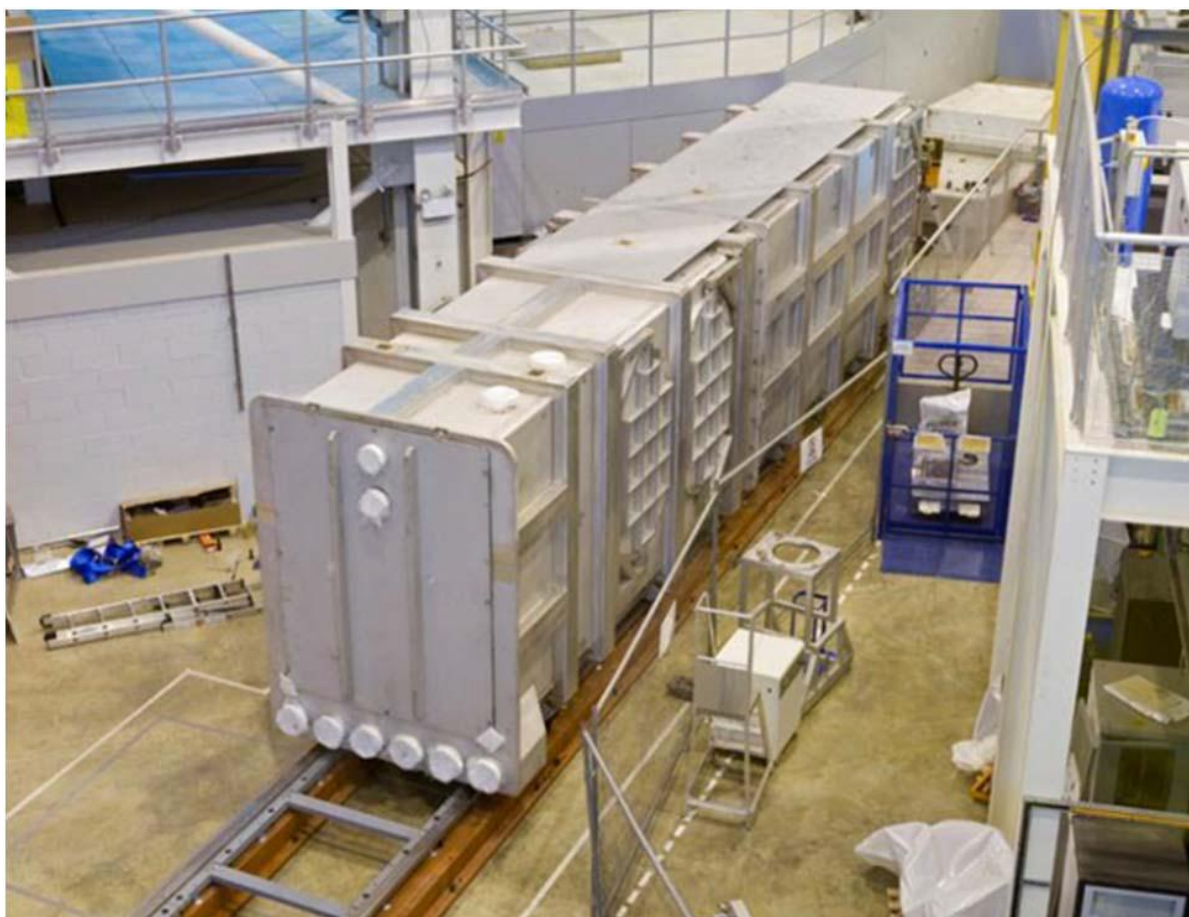
The ZOOM tank after welding. Zoom is one of 4 new instruments on Target Station 2 of ISIS. Photograph courtesy of STFC
