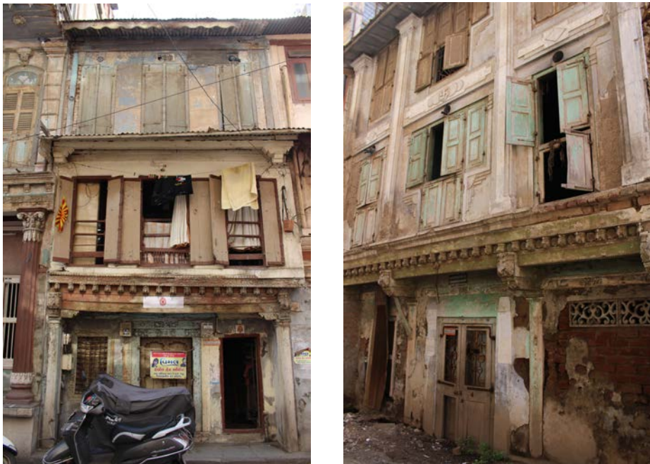
Figure 14 & 15: Dilapidated heritage buildings (Rander)
