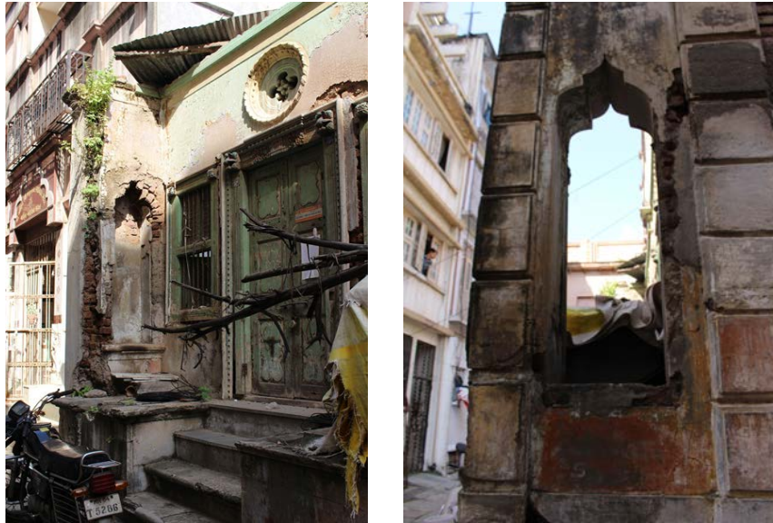
Figure 16 & 17: Heritage buildings in need of restoration (Rander)
