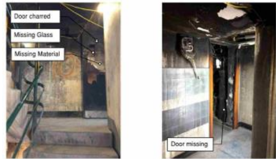
Figure 6: Damaged or missing flat door
