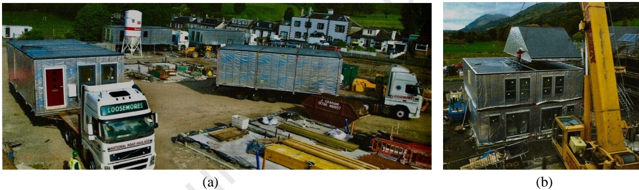
Fig. 3. (a) The modular units are delivered to the site by lorries to reduce both the cost and time of the construction phase in the UK. (b) The modular units are assembled on site within 24 h, including fully fitted interior finishes. Image Credits: Tigh Grian Ltd (Scotland).
