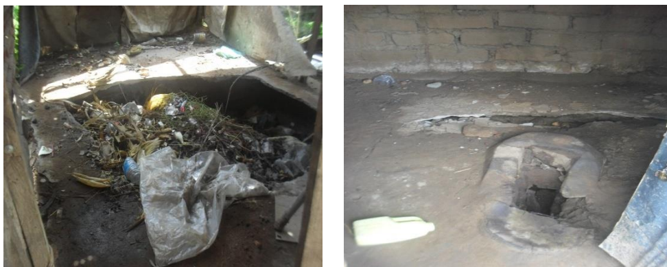
Collapsed latrine in Gumbo which now serve as a household rubbish dump; Collapsing latrine in Lologo.
