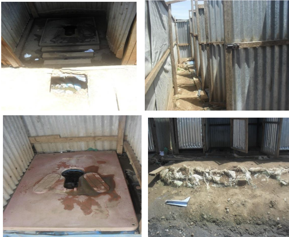
Clockwise: Plastic bottles in a pit latrine in PoC 1; Damaged locks of a latrine block in PoC Site 1; Removed cover of a plastic slab; Stump of a dismantled privacy screen.
