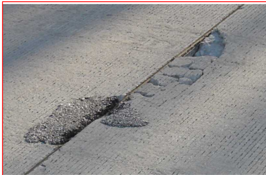
Figure 2.29 Spalling (Source: Jung, et al., 2008)
