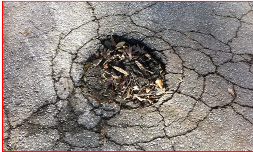
Figure 2.17 Potholes (Source: Neal, 2013)
