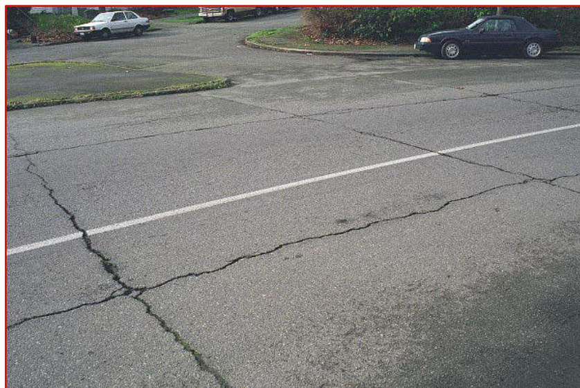
Figure 2.15 Block cracking (Source: Mathew, 2015)
