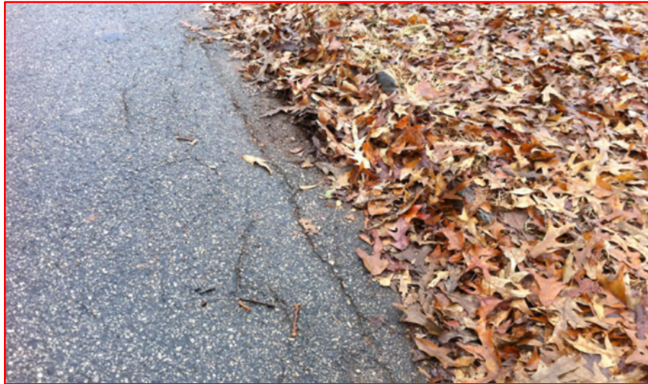
Figure 2.16 Edge cracks (Source: Mathew, 2015)
