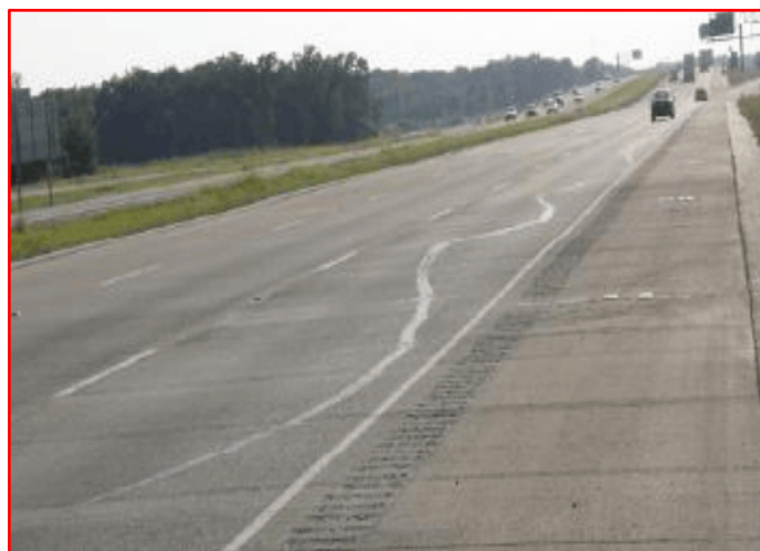
Figure 2.28 Longitudinal cracks (Source: Jung, et al., 2008)
