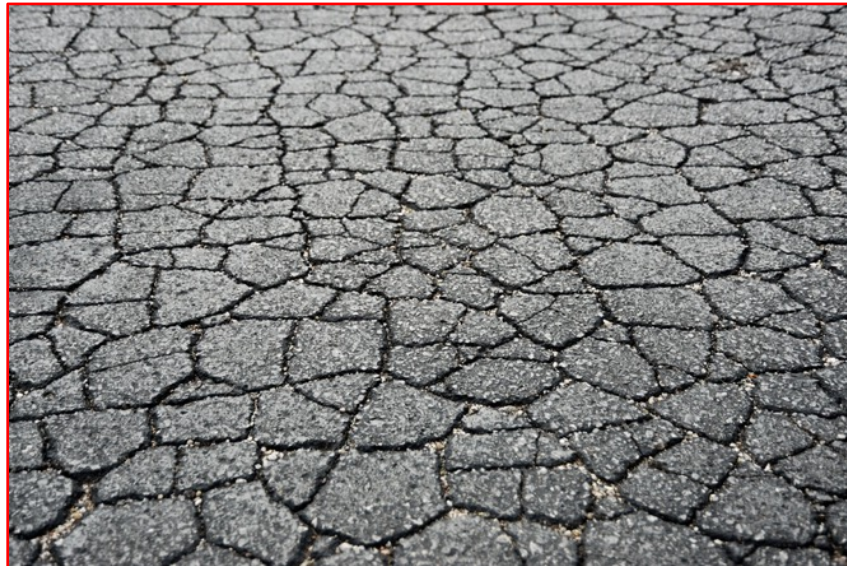
Figure 2.14 Alligator cracking (Source: Mathew, 2015)
