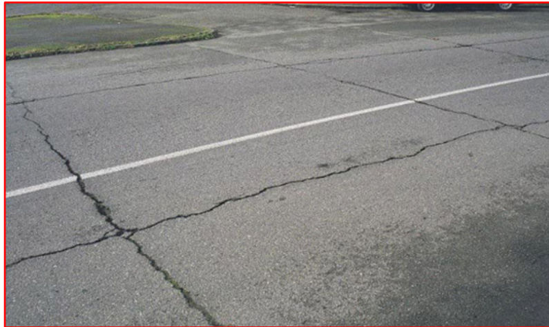
Figure 2.27 Joint cracks (Source: Neal, 2013)
